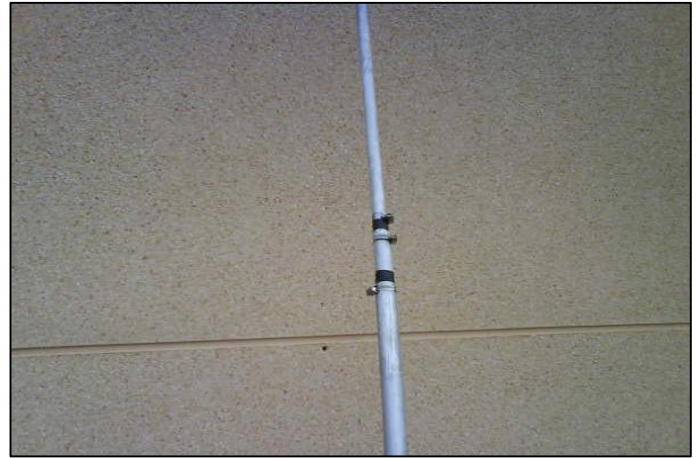
Photograph showing the Jubilee pipe clips use to secure the sections of aluminium tubing together.
